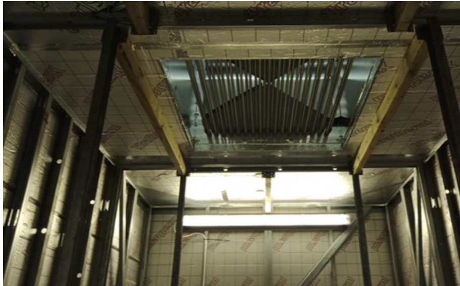
Figure 3 Wind tower and heat pipes viewed from within the test room.
