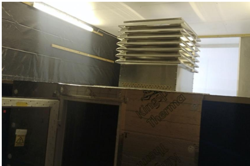
Figure 4 External view of the wind tower.
